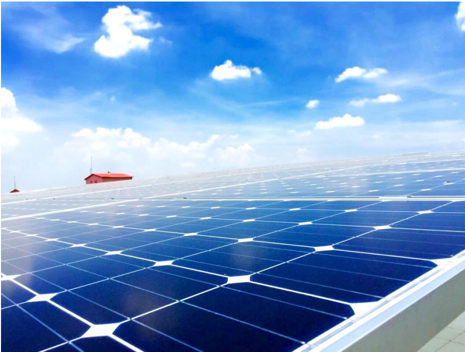
※ Our solar PV system in Miaoli, Taiwan
